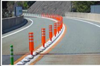
Orange color has a good visibility but rubber bar cannot prevent car from jumps out
